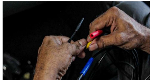
STEP 16 :- DISCONNECT ALL THE CAMERA CABLES
